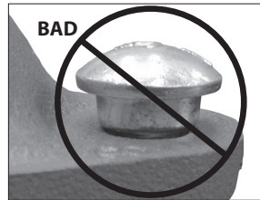
OVAL NECK OF BOLT NOT SEATED PROPERLY
