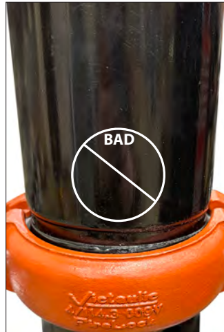
PHOTO 3 (UNACCEPTABLE) – HOUSINGS' KEYS NOT ALIGNED WITH PIPE GROOVES
