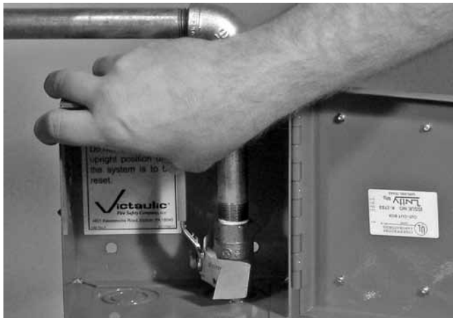
20. Close the manual pull station.
