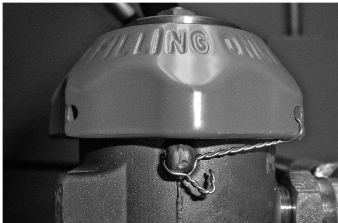
Cylinder valve shown above is safety wired in the closed position
