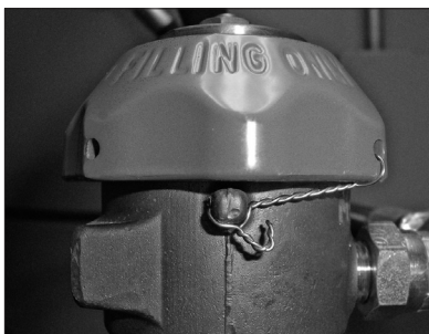
Cylinder Valve shown is safety wire tied in the closed position
