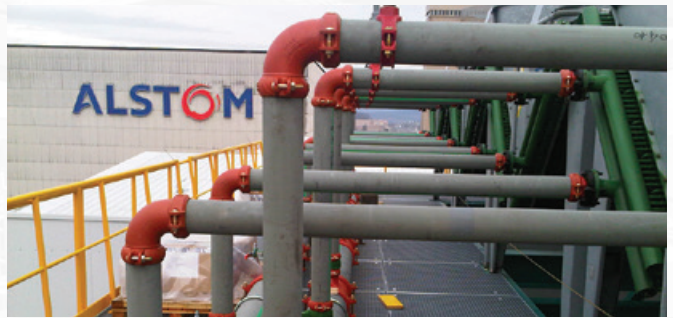
Alstom Birr Power Plant
