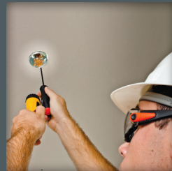
Secure sprinkler in bracket
