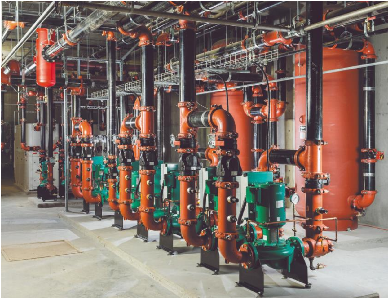
Mechanical room inside a commercial building featuring Victaulic pipe couplings, valves, and elbows.
