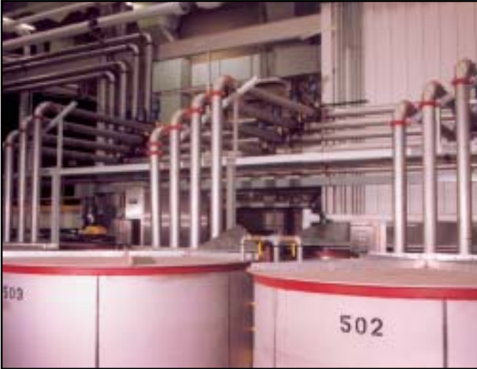
The Victaulic grooved system is ideal for piping galleries. By providing a union at every joint, the Victaulic system allows you easy access to the system for maintenance and changes.
