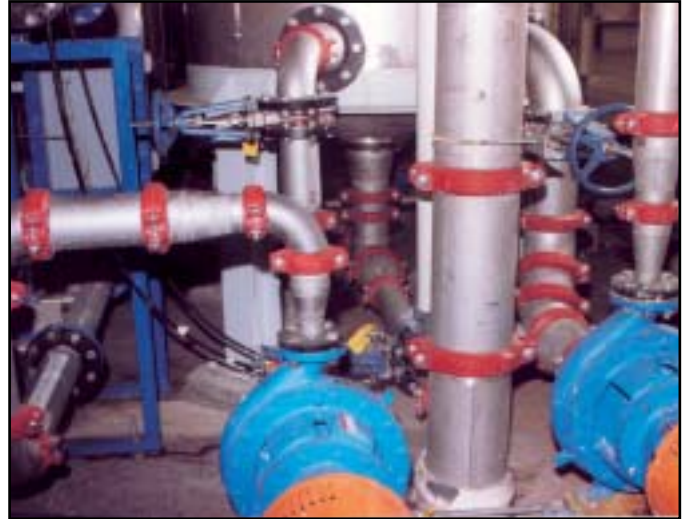
Restricted spaces, such as this mechanical room, are another example of where the grooved system can decrease your costs. Since couplings can be rotated and oriented in any direction, installation is much faster and easier. There are no two-holing problems as with flanged components, or smoke and flame concerns as with welding.
